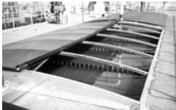
A retractable, structurally supported cover system is used to cover the influent channel and primary clarifiers.
