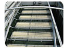
A membrane reactor tank opened for inspection.
